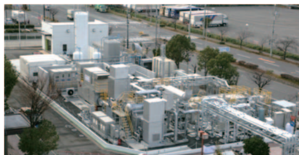
a) Hydrogen fueled power generation plant
