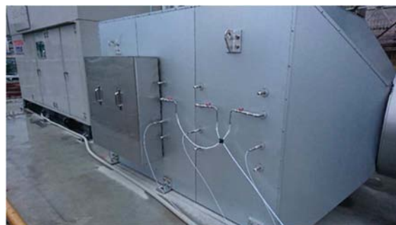
Fig. 6 NOx removal unit (SCR)
