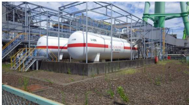
Fig. 4 Ammonia supply facility
