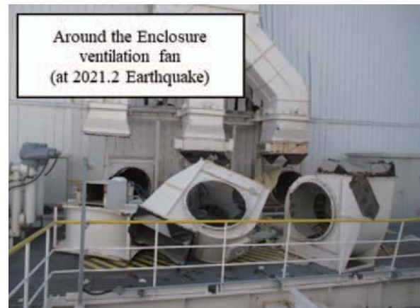
Fig. 5 Damage situation in Sendai thermal power station
