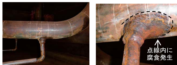
Fig. 5 Corrosion and Crack around Nozzle
