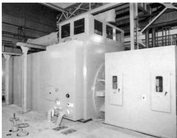
Fig. 9 Generator for gas turbine
