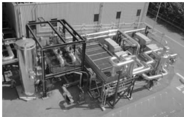
Fig. 14 Exterior view of air cooling system
