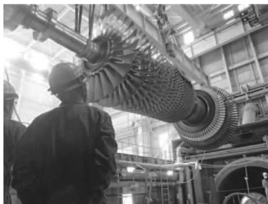
Fig. 15 A periodic inspection of gas turbine
