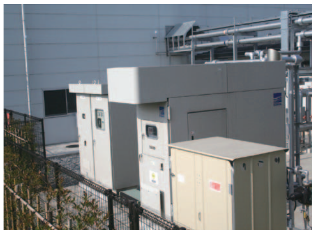
Fig.11 Micro gas turbine
