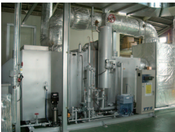
Fig. 3 Heat recovery steam generator
