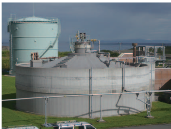
Fig. 2 Gas Holder and Digestion Tank
