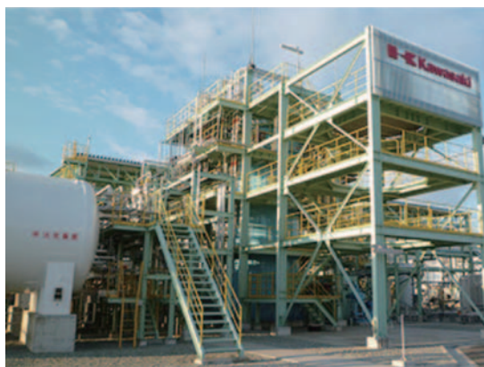
Fig. 3 Liquid hydrogen production test plant
