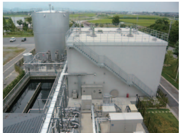
Fig. 9 Methane fermentation tank
