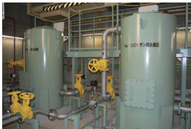
Fig. 3 Siloxane Removal System
