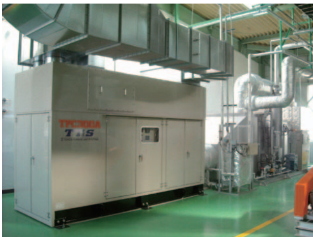
Fig. 2 Micro gas turbine Generation package Unit
