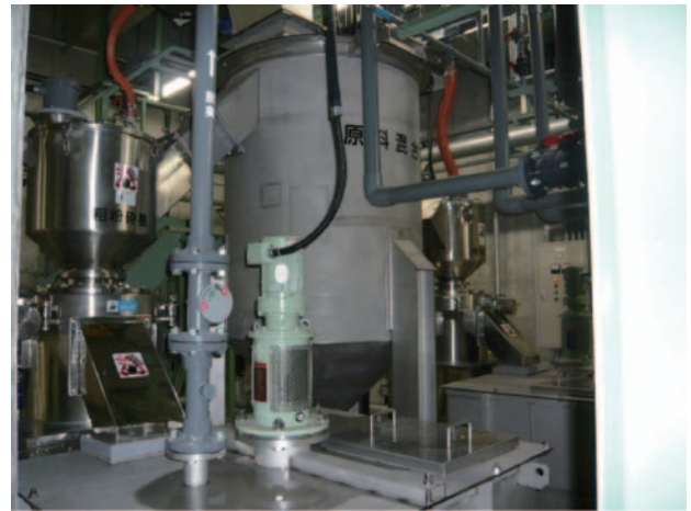
Fig. 8 Mixing tank・grinder
