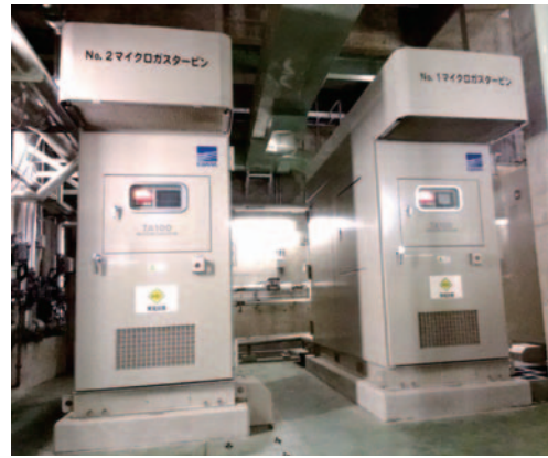
Fig. 5 Micro Gas Turbine
