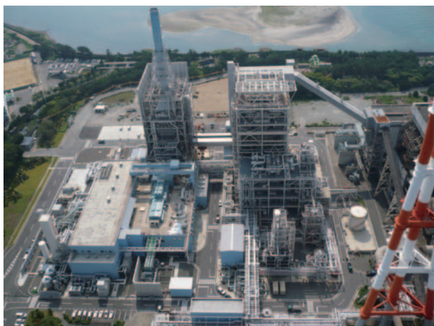
Fig. 10 Bird's-eye view of IGCC demonstration plant
