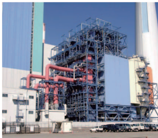
Fig. 7 De-sulfurization system of Isogo #1
